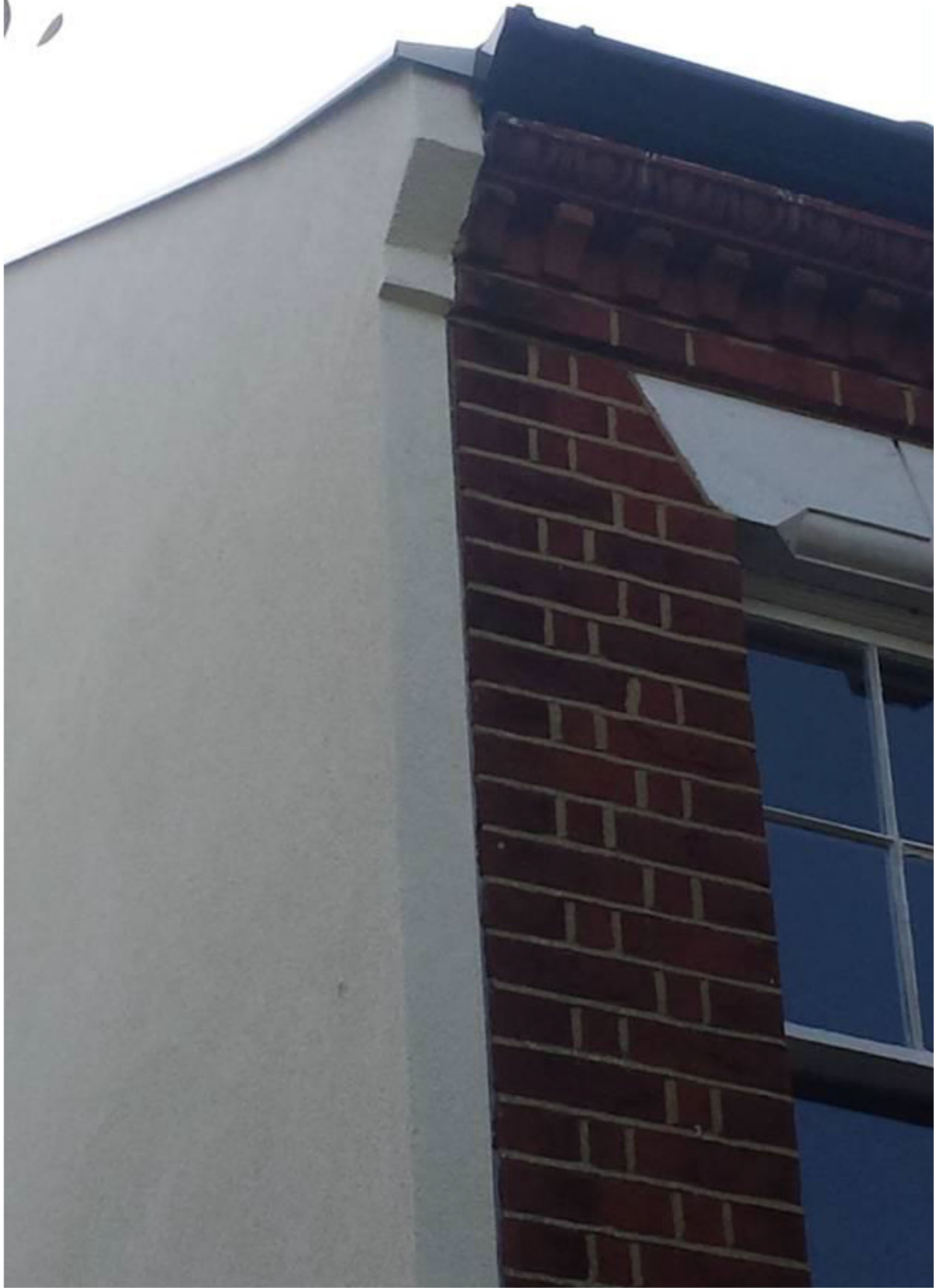
Elevation showing detail of eaves, flashing and capping at front of property
