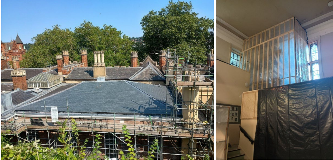
The new Courtroom roof and repairs underway in the Costume & Textile store
