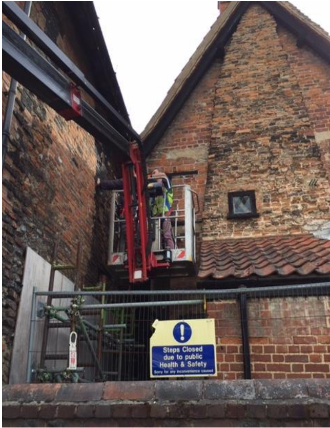
Photo 1 - North elevation (looking from River) of 22-24 Elm Hill (right building) and 26-28 Elm Hill (left building) – showing the extremely narrow gap between the two buildings (into which the flue was unlawfully inserted) and the damaged and structurally compromised west wall of No.26-28.
