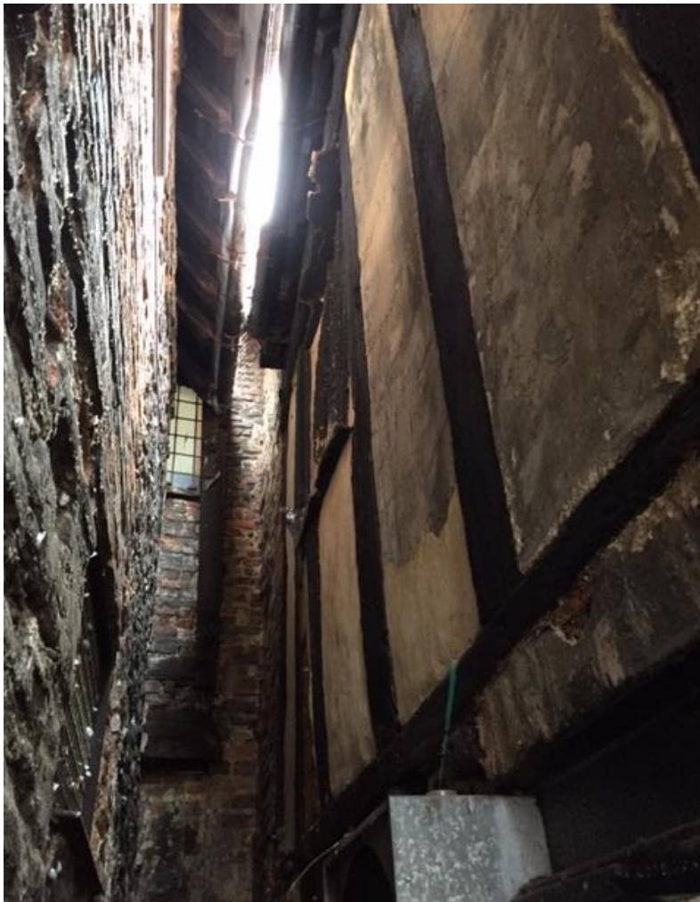
Photo 2 – On right of picture – Timber framed east elevation of the Stranger’s Club with the unauthorised extract unit (fire risk) located directly below the C16th timber framed jetty beam. On left of picture - West elevation of 26-28 Elm Hill severely damaged by years of moist fatty flammable emissions in the enclosed gap between the buildings.
